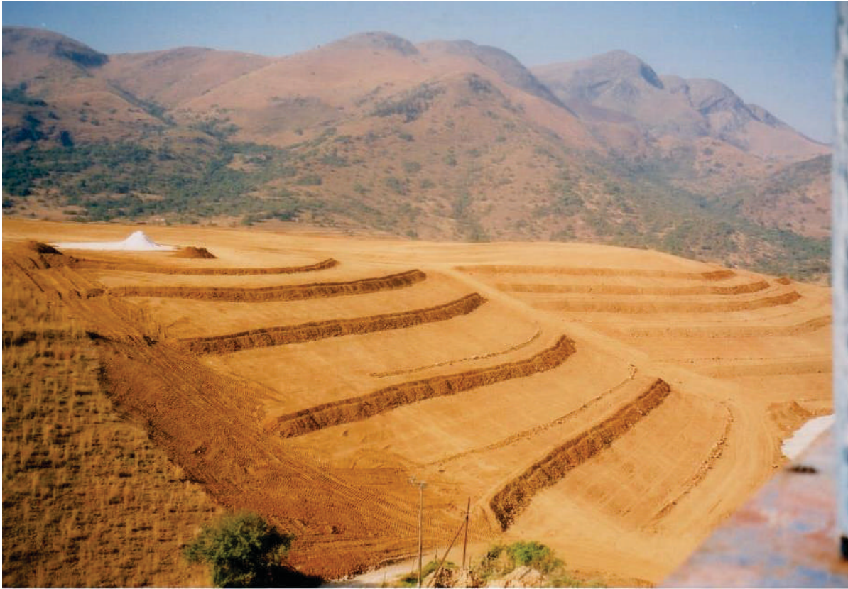
Covering and shaping the Msauli mine dump in accordance with rehabilitation requirements
