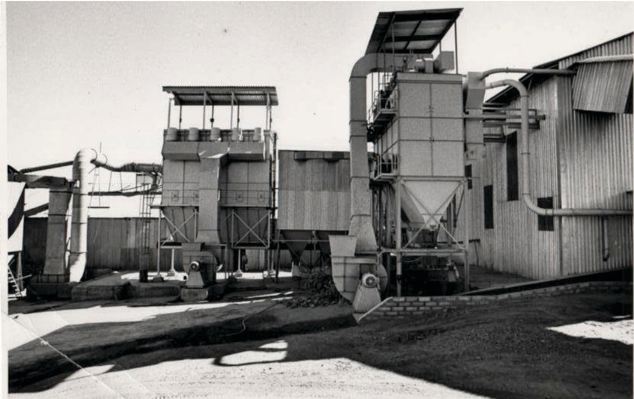
Dust extraction units attached to the existing milling structures, as seen at the Riries mill
